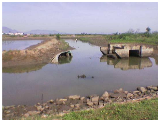
Figure 5. Remain of a destroyed bridge at Syah Kuala
