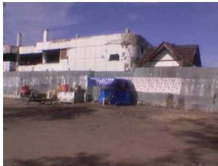
Figure 3. Tsunamis destroyed buildings still remains intact. Some of them (middle) are inhabited illegally.
